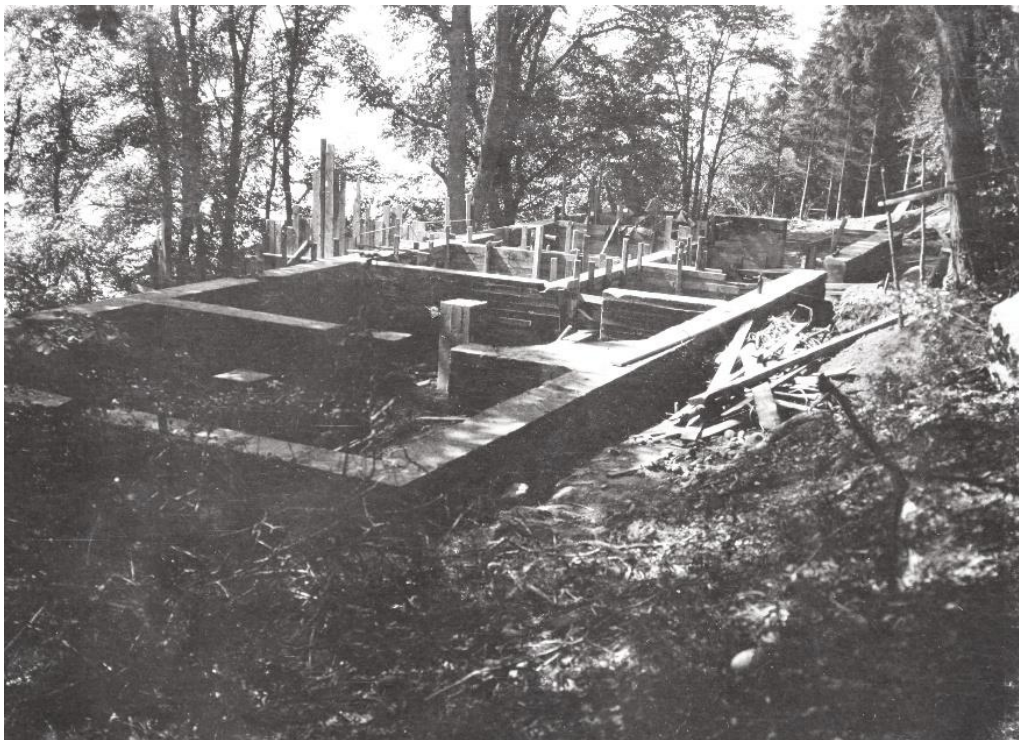
The Strand building site, summer of 1910. From the Ellen Key archive, Royal Library, Stockholm
